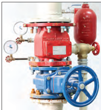
Valve configuration on a Wet Pipe system
