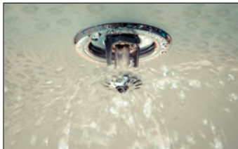
Discharge might occur if a sprinkler head is accidentally overheated or damaged
